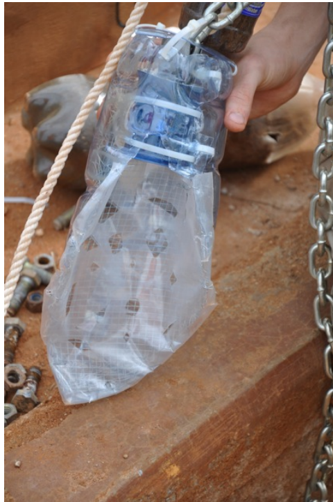
Figure 9: The "Skirt of Salvation," just before it was lowered into the well to settle onto the top of the pipe and guide the Harpoon of Death into the pipe. [June 17]
