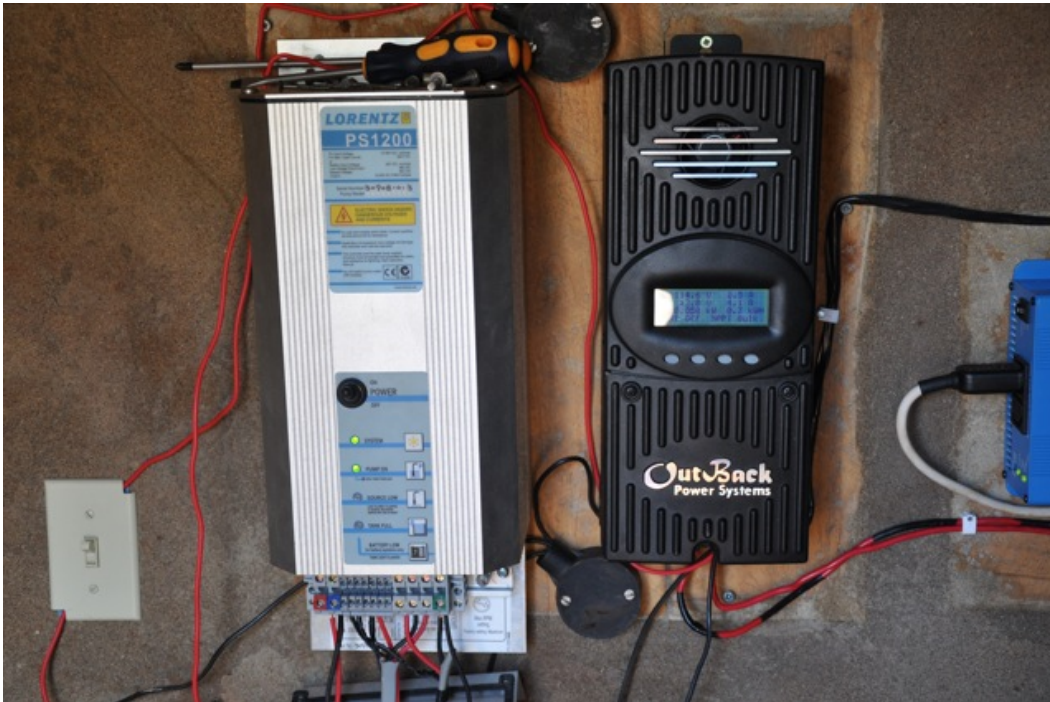
Figure 18: Pump controller and charge controller. [July 13]
