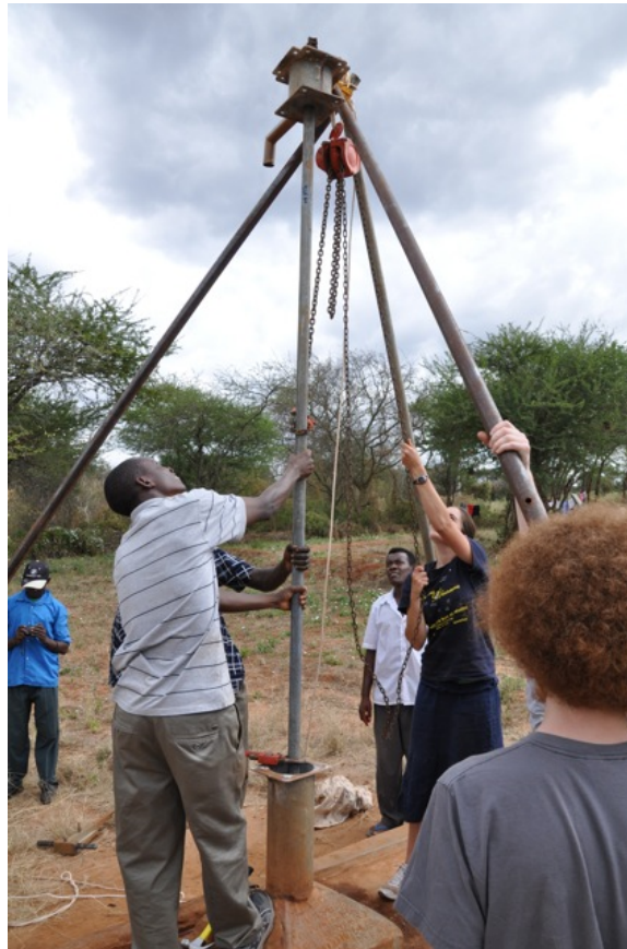
Figure 4: Raising the old pump. Note how the flange with the spigot appears to be impacting the rope that holds the chain hoist. [June 13]
